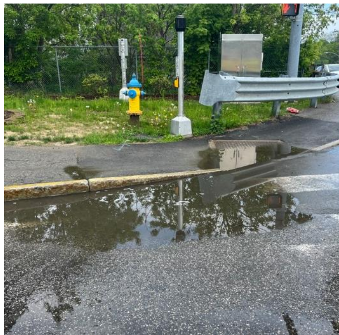
Figure 21 – Drainage issues at Southeast Corner of State St and North Main Street.
