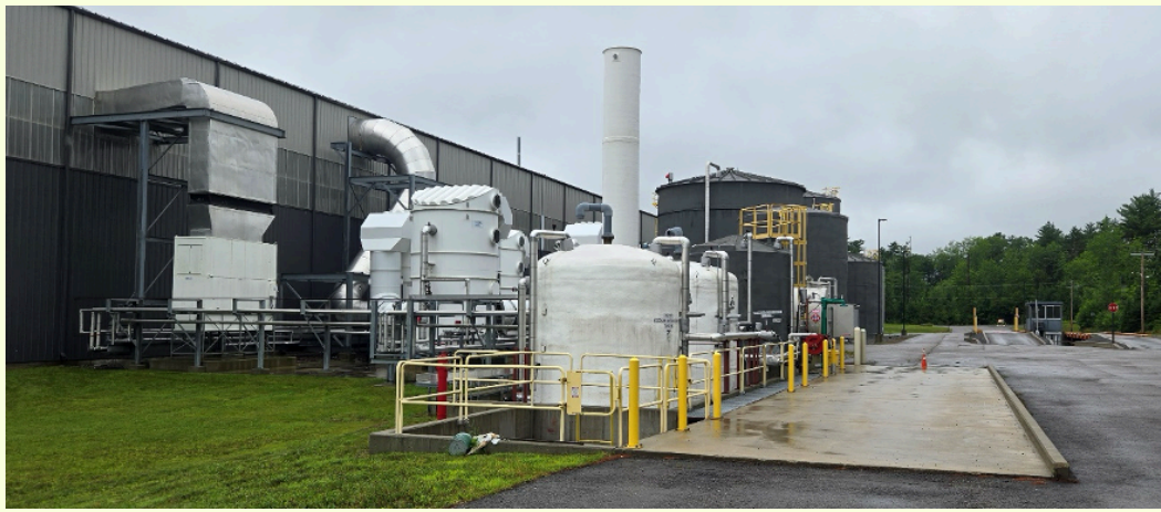
Odor abatement air scrubber system in the foreground; anaerobic digester in background
